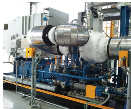
Boil Off Gas Compressor for LNG Terminal
