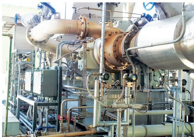
Steam Compressor for Mechanical Vapor Recompression
