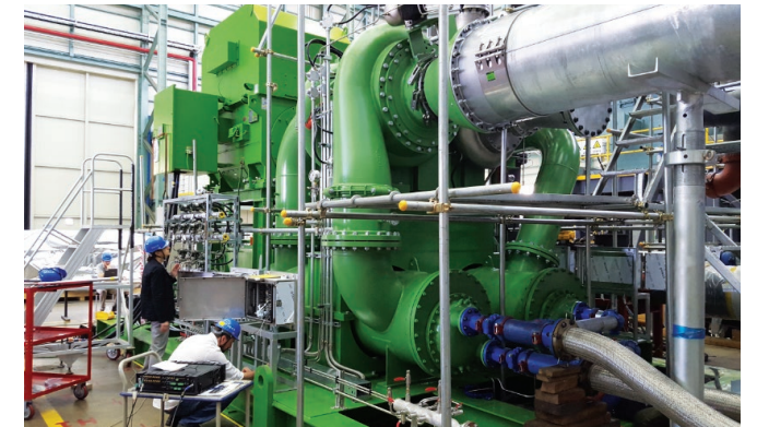
Compressor for Hydrogen Peroxide(H 2 O 2 ) Process
