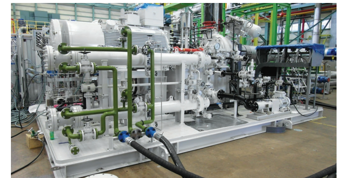
VRU Compressor for Offshore artificial island
