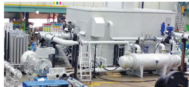
Fuel Gas Compressor for Cogeneration Plant
