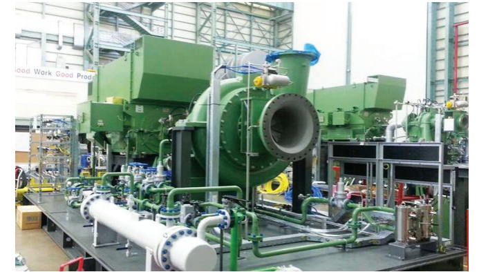
Process Air Blower for Carbon Black
