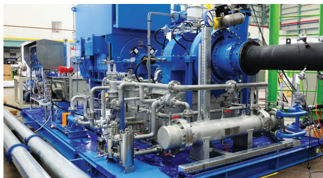
Process Gas Compressor for Fertilizer Facility
