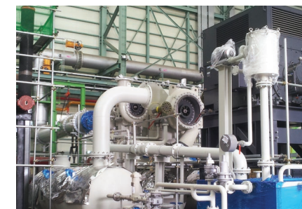
Air Compressor for Air Separation Plant
