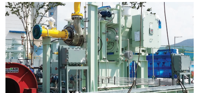
Fuel Gas Compressor for Combined Heat & Power Plant
